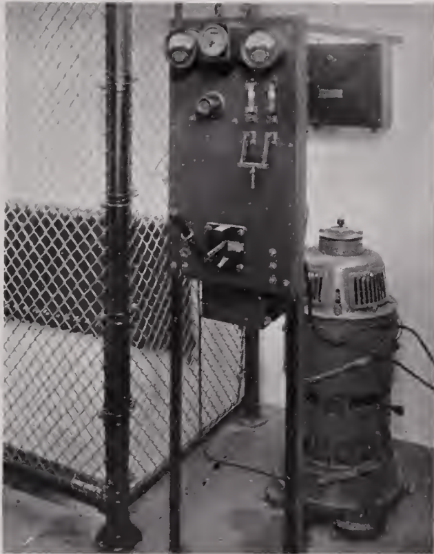
BATTERY CHARGING GENERATOR
